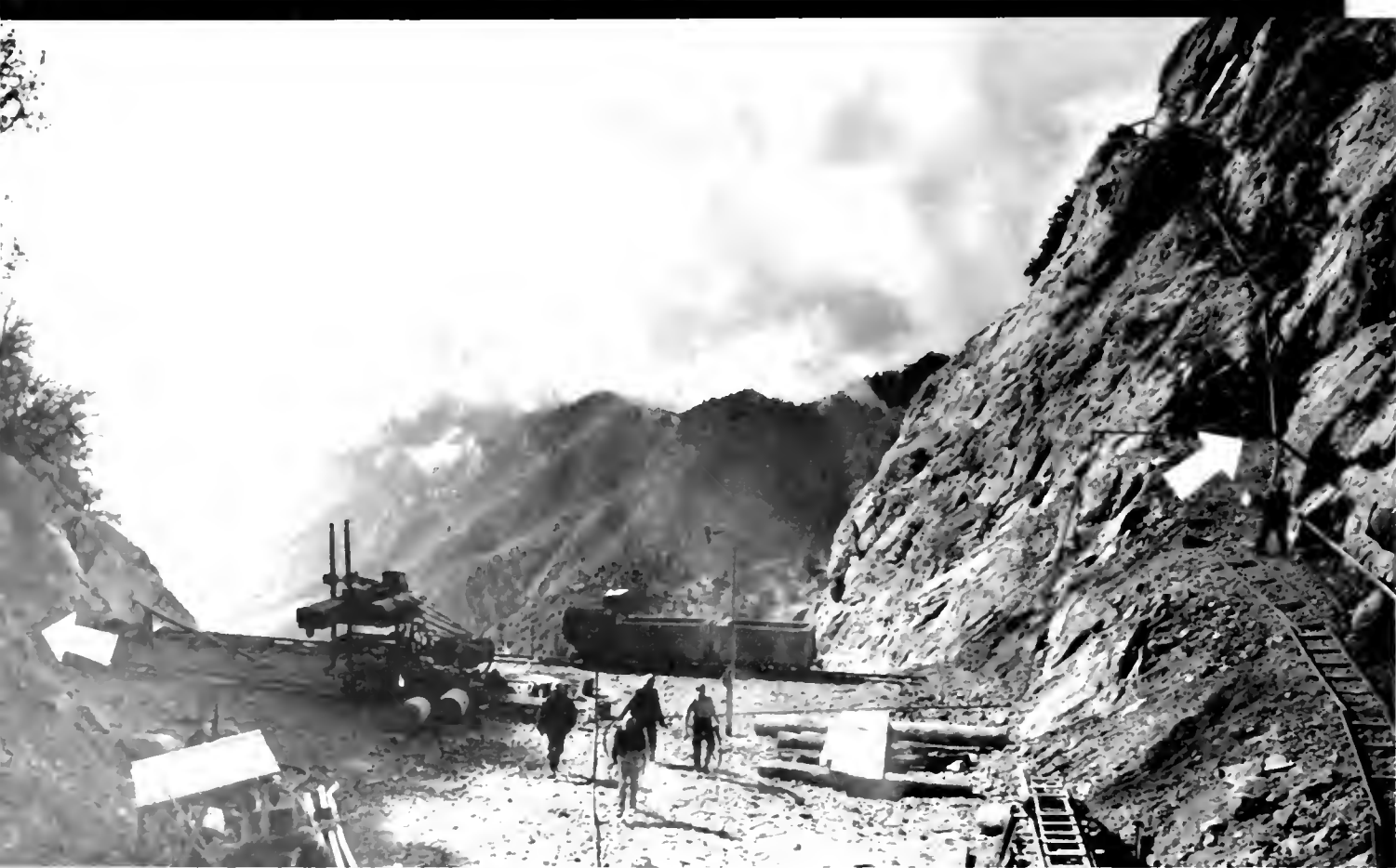
Arrows point to 2 tunnels separated by only 87 feet of highway being bored through Mt. Williamson on Angeles Crest Highway.
